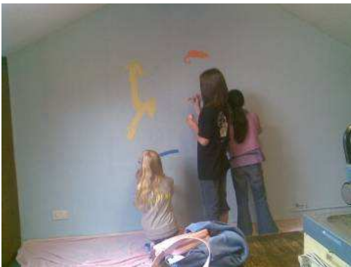
The crèche room gets a makeover as Red Group starts to paint the mural
